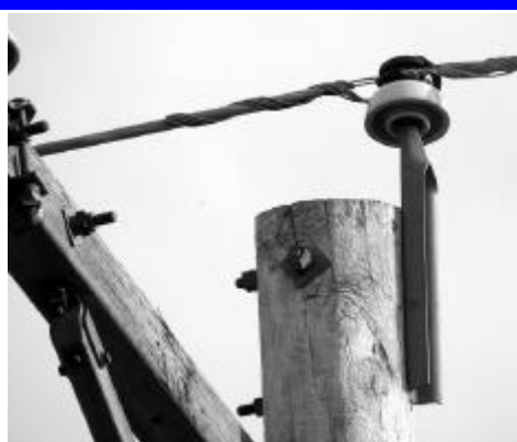
This example of ice storm damage was found in the Holdrege region early this spring.
