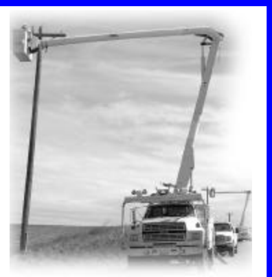
Contractor crews worked near Norman in March rebuilding miles of distribution line, essential for this summer's irrigation load.
